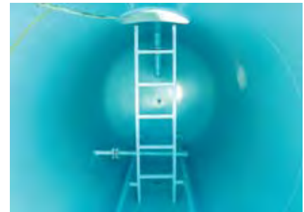
The vessel was coated with Devchem 253 in our shop. Complete inspection followed, with QA/QC reports given to customer.
